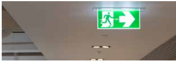
Photo: Exit sign
