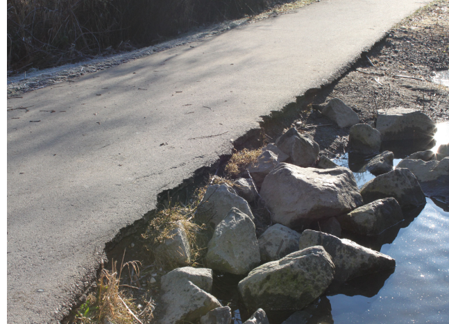
2 Erosion and Asphalt Eroding Along Pathway
