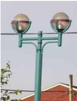
existing twin head Pace luminaire
